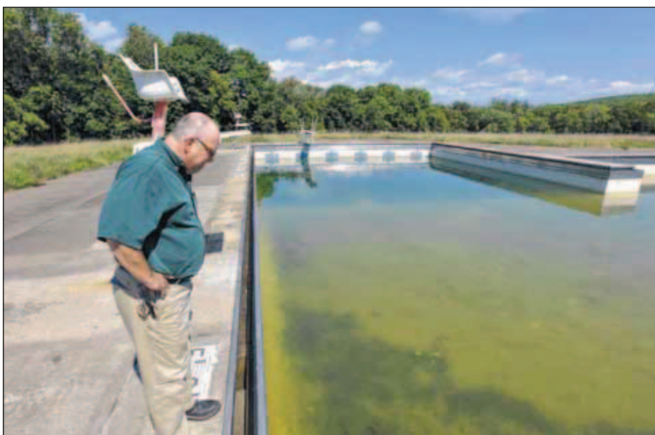
Photos by Pete G. Wilcox | Times Leader Nick Lylo, district forester for Bureau of Forestry's Pinchot Forest District looks at the pool in Moon Lake Park. The structure will be filled in and this fall.
