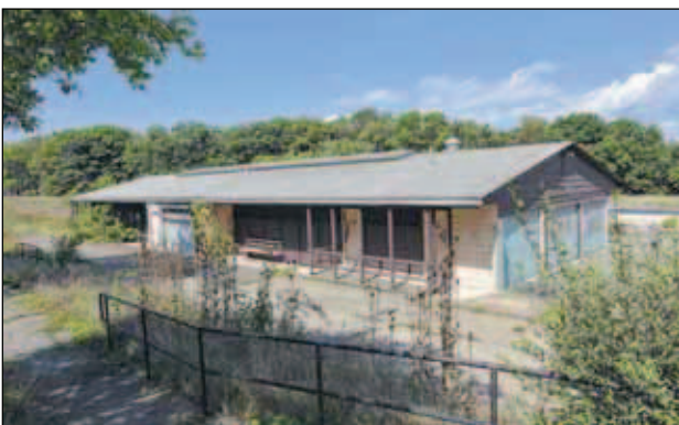
The pool house at Moon Lake Park is boarded shut after vandalism damaged the structure. The building will be demolished this fall.
